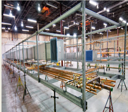
The MEP system compenets are assembled in a prefabrication shop with a controlled environmnet
