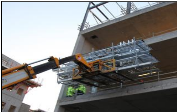
Figure 20 The installation process of the MEP system modular. Image courtesy of www.globaloff-site.com
