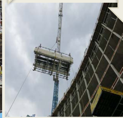
Different euipement are used to place the MEP system compenets to their final location
